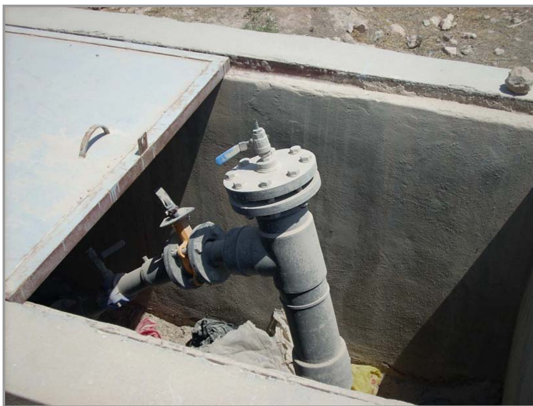
Figure 4 One of the 96 wells at the landfill site. The wells are protected by a concrete box and covered with a steel plate.
