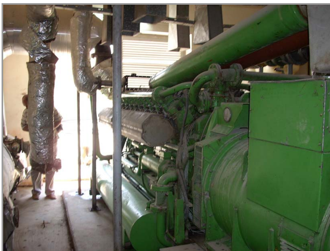
Figure 2 The 1-MW Jenbacher biogas engine installed by Farmatic.
