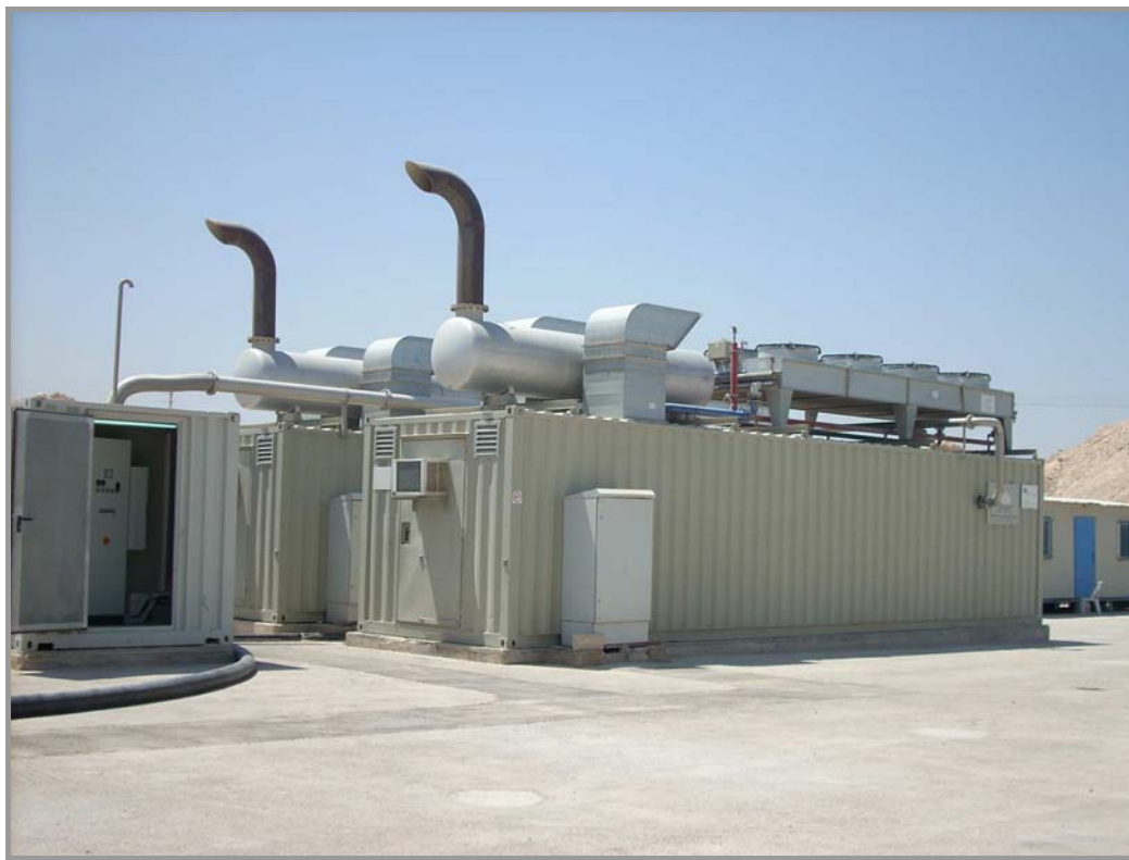
Figure 3 The two 1.25-MW biogas units added to the Ruseifah plant under the UNDP/JBC Phase-2 expansion project.
